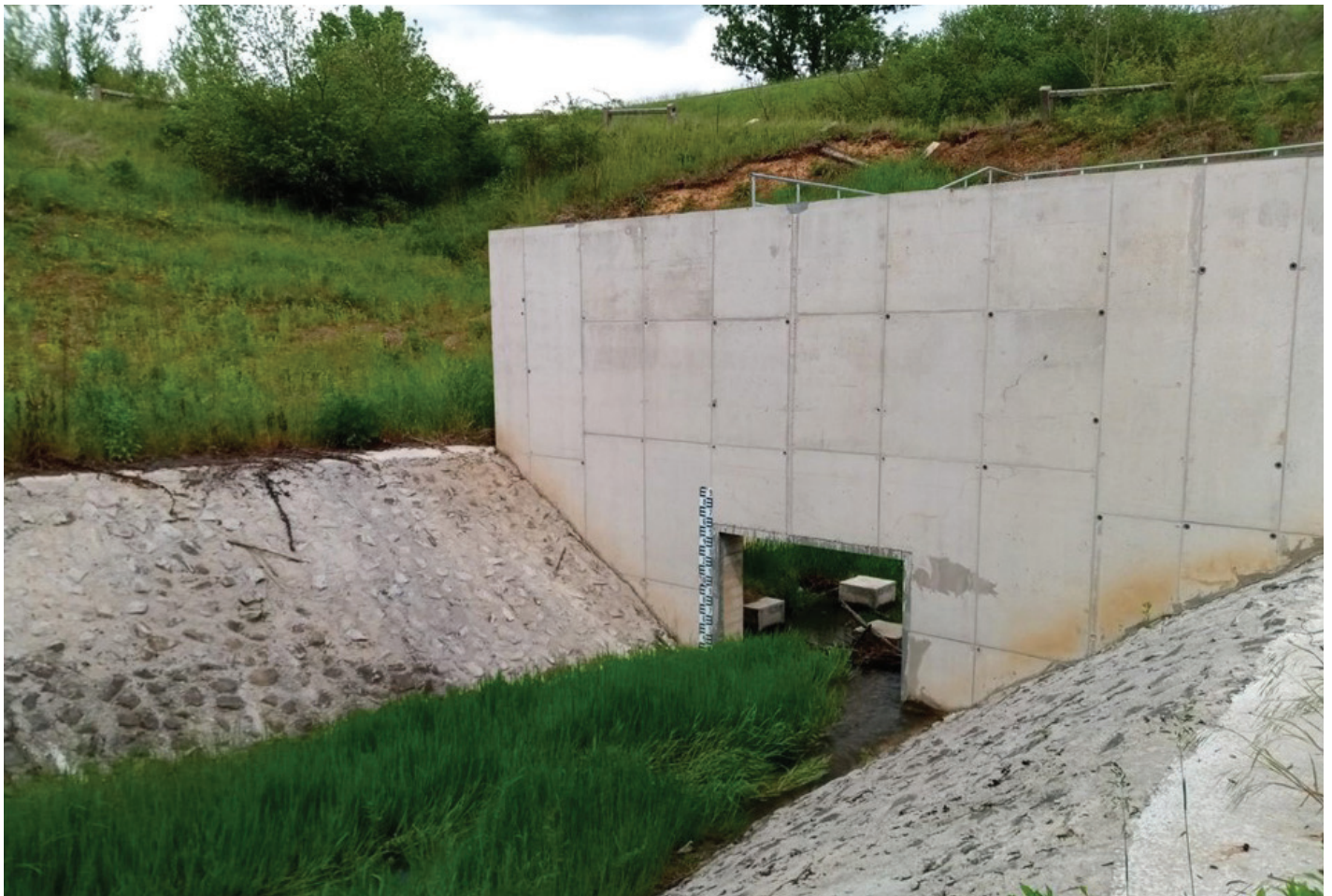
Figure 28 Road No. 2 crossing of the Hévíz-stream with an inappropriately sized culvert
